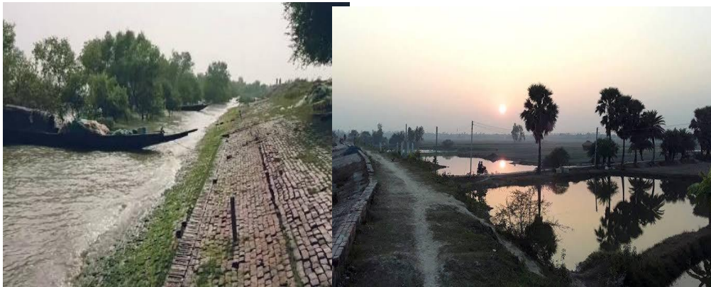
Fig: Dam contraction
