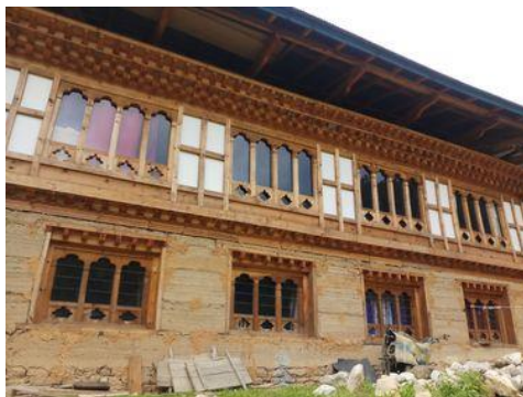
g. Composite rammed earth (ground floor) and wattle and daub (first floor)
